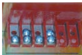
Secondary terminal box (2 secondaries and grounding screw)
